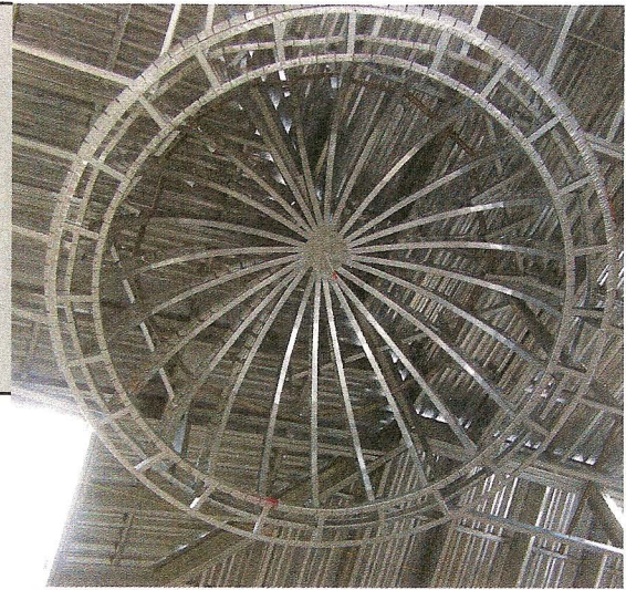
One of the things he likes best about building with steel is its design flexibility, and says it is easy to frame barrel ceilings, domes (pictured here) and other details with steel.
